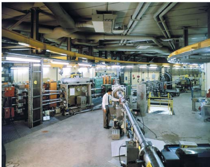
Fig. 10. PS Booster seen from the injection/ejection region
